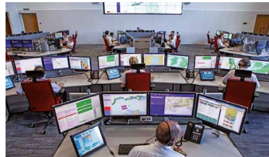
Centrale MRCC (Maritime Rescue Coordinator Center) Portland UK.
